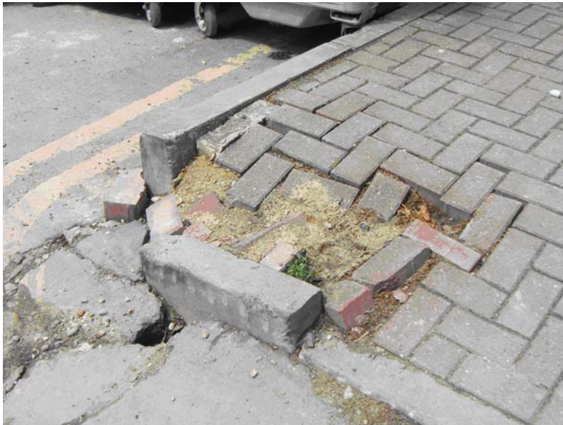
A trip hazard: This damage was caused by delivery vehicles running over the corner of a curb. Have you seen damage like this on your estate? Report it to Peabody Direct on 0800 0224040
